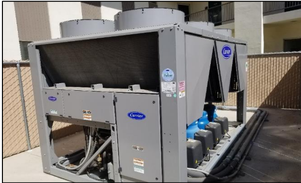
New 100-ton central chiller
