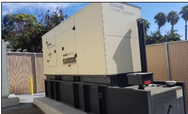
A new vivarium generator provides more protection for research programs
