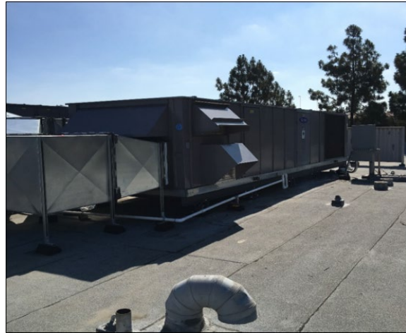
New Air Handler at 6386 Alvarado Court
