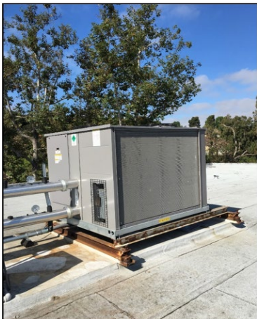
New Chiller at 6330 Alvarado Court
