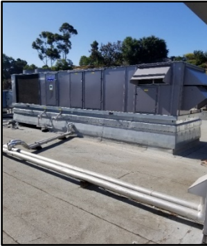
6386 Alvarado Court (Roof) – New air handler #3
