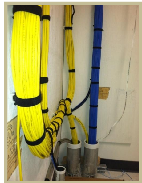
Category 6 cabling enhances IT bandwidth at Alvarado Medical Center
